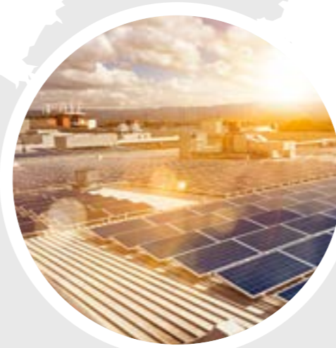
3. SHELLHARBOUR SHOPPING CENTRE, NSW Module: CS6P-P Power generation: 1.2 MW
